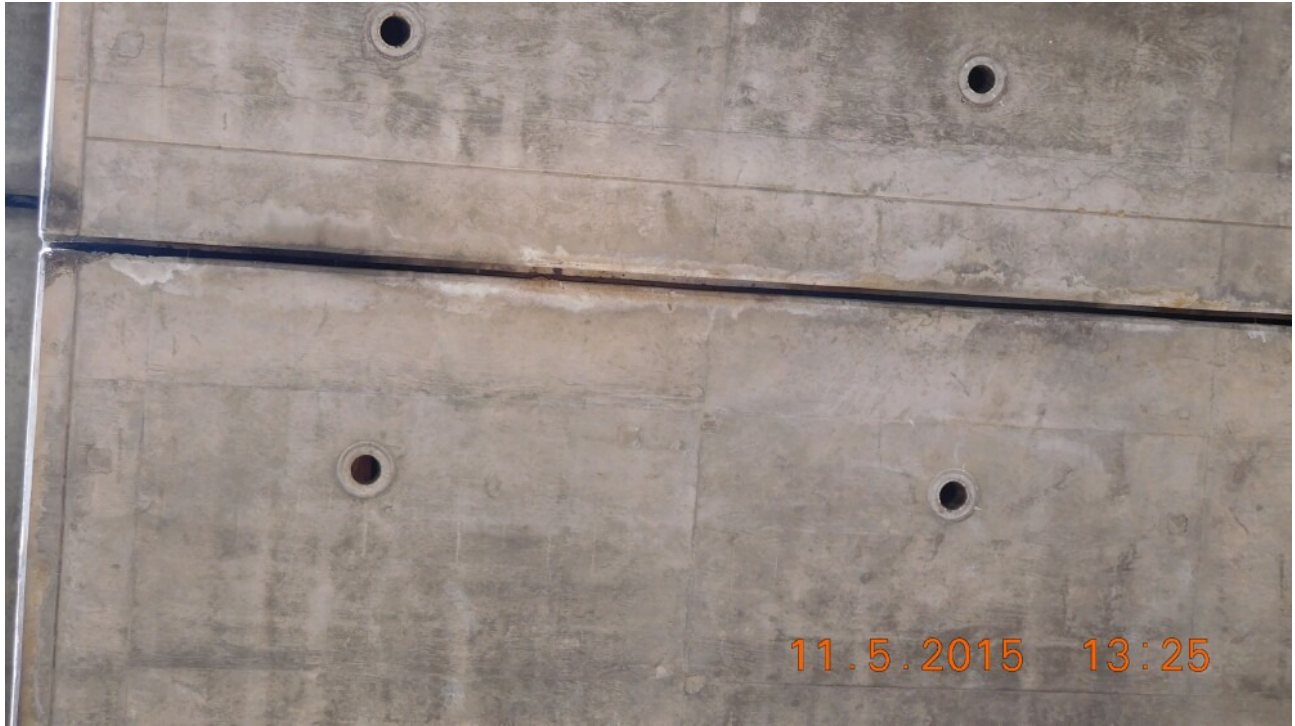
Figure 7. Roosting activity in expansion joints. Unknown whether bats are entering girder interiors through weep holes, but evidence of use by birds was present.
