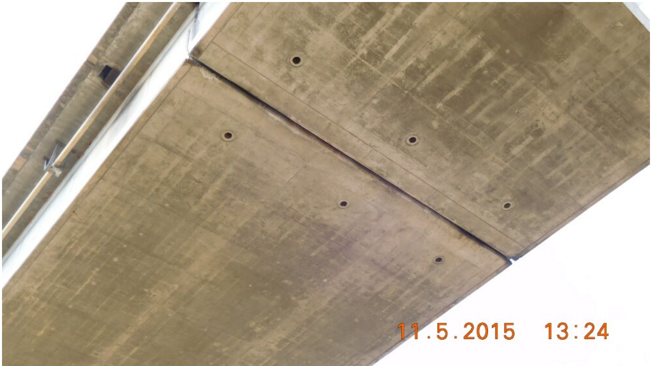
Figure 8. Roosting activity in expansion joints. Unknown whether bats are entering girder interiors through weep holes, but evidence of use by birds was present.
