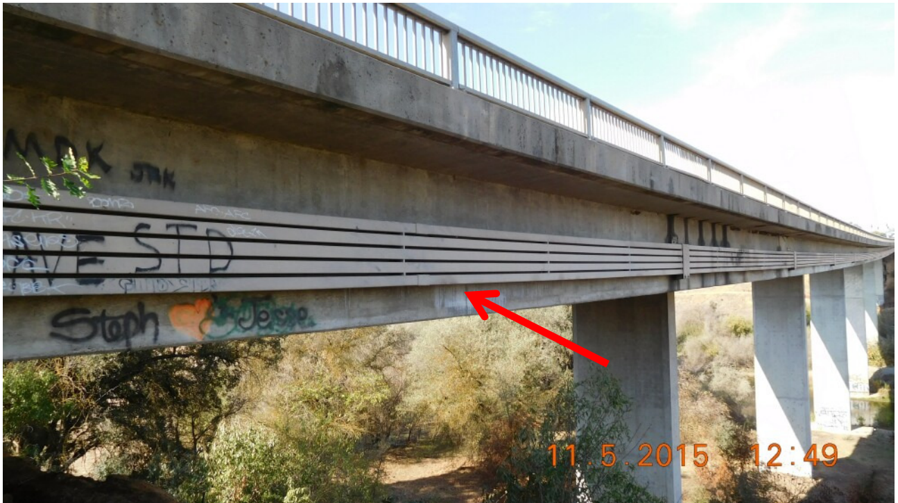
Figure 2. View from south end of bridge. Dead bat observed in roost crevice behind utility channel assembly at arrow.
