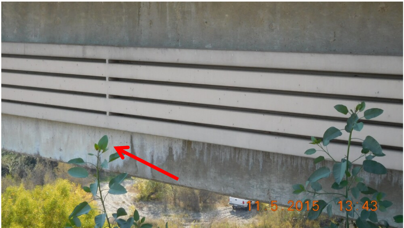
Figure 3. Extensive areas of bat urine staining and bat fecal matter on soffit behind, beneath, and on utility channel assembly.
