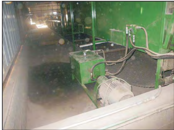
Photo 11: Hydraulic oil leak at packing machinery.
