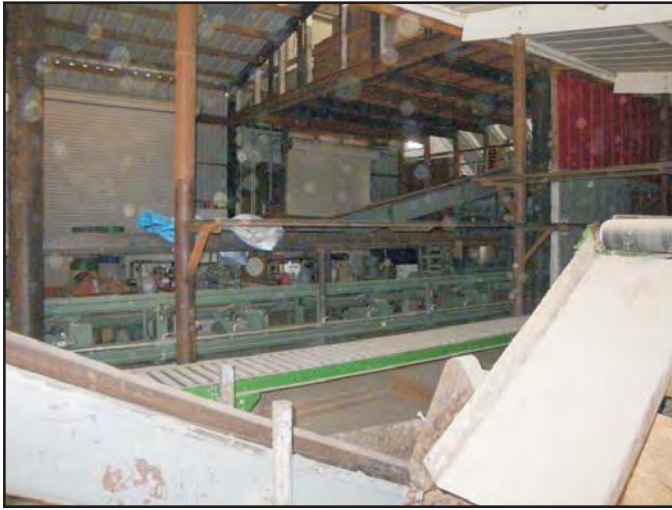
Photo 10: Produce packing machinery along south wall inside western portion of barn/packing shed.
