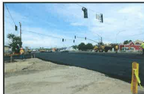
Kiernan intersections were raised to the new bridge elevation at the completion of Stage 2.
