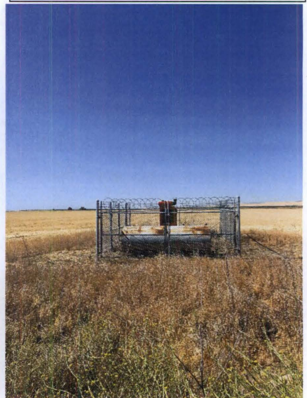
Figure 7 (below): Well 6/8-20G is newly fenced and has a new motor connected.
