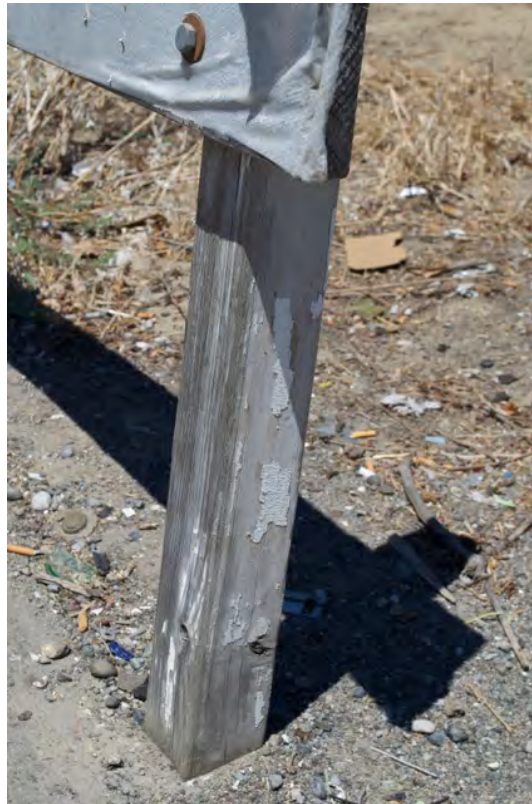
Photo 8 – Chipping and peeling paint on wooden guard rail.
