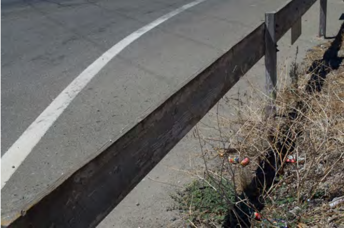
Photo 9 – Back side of wooden guard rail showing chipping and peeling paint.
