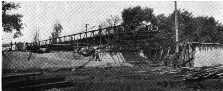
Construction Photo of Pajaro River Bridge: This Photo Shows A Canticrete Bridge With Its Trusses, Before Concrete Encasement Source: The Architect and Engineer of California, 1919. Digitized By Google.
