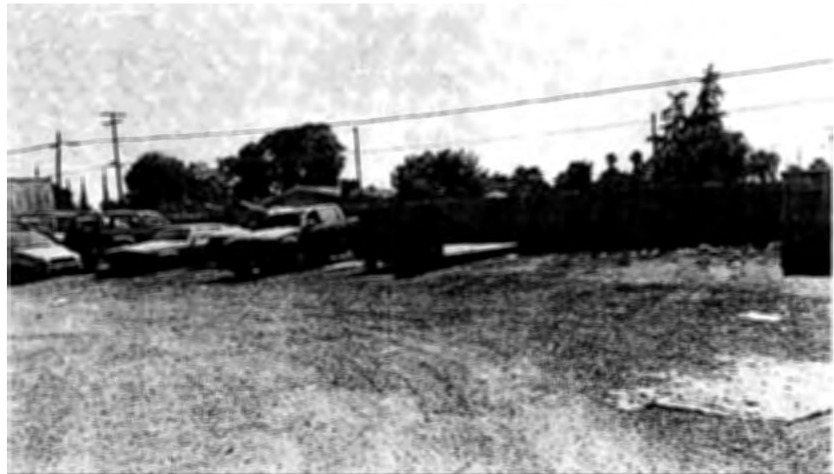
Looking east to property line by Bystrum Road. The ten foot high wall, landscaping, storm drainage system and paved floor not installed.
