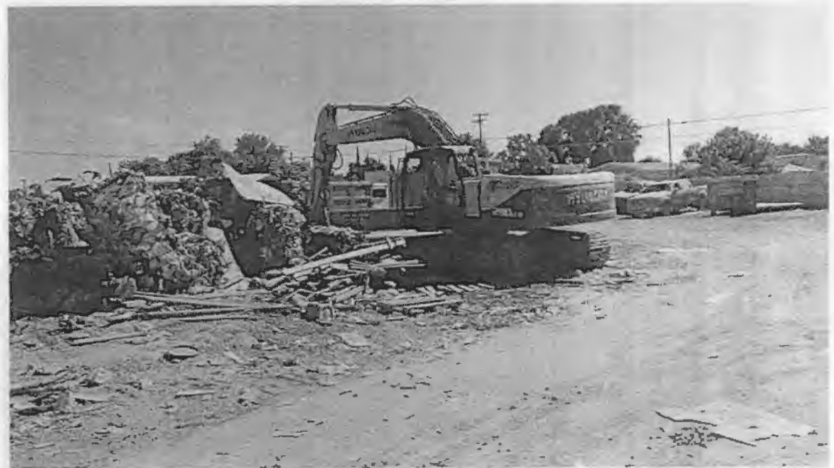
Looking Northeast mid property. All loading and unloading by excavator to occur west of "tin pile."
