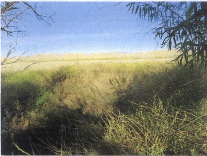
Figure 12 (left): Pickup drain looking over fields that is full of vegetation.
