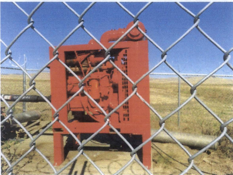
Figure 11 (left); New motor placed on existing well to make it operational. This well was also fenced in this year to cut down on vandalism.
