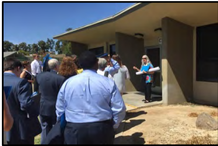
BHRS Director Dr. Madelyn Schlaepfer shows the CSU under construction to members of the MHSOAC during their visit to Modesto on August 27, 2015.
