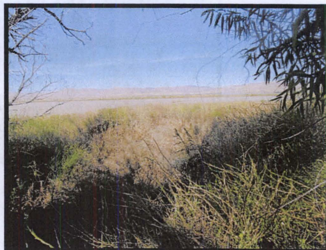
Figure 14: Pickup Ditch, with excessive vegetation blocking culvert.
