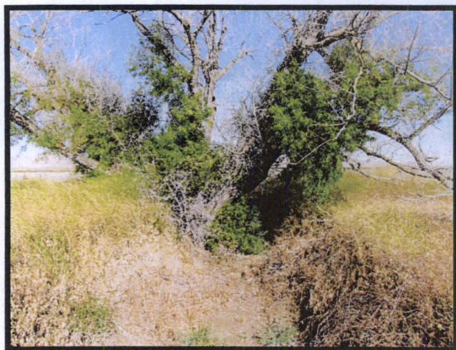
Figure 13: Pickup Ditch, significant vegetation and sediment build up blocking culvert.
