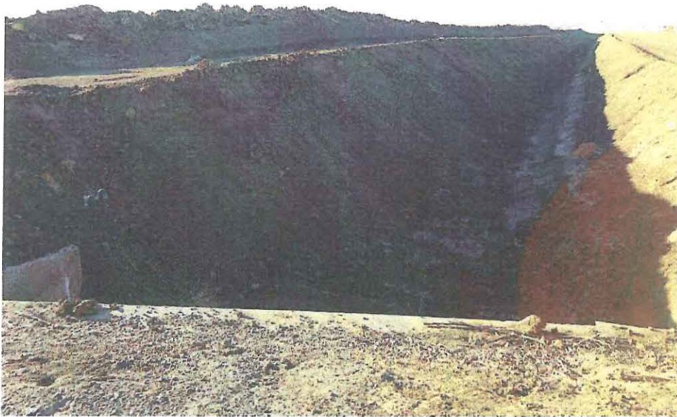
Figure 9. Little Salado Creek has recently been cleaned out; there is still some congestion in culvert under the road
