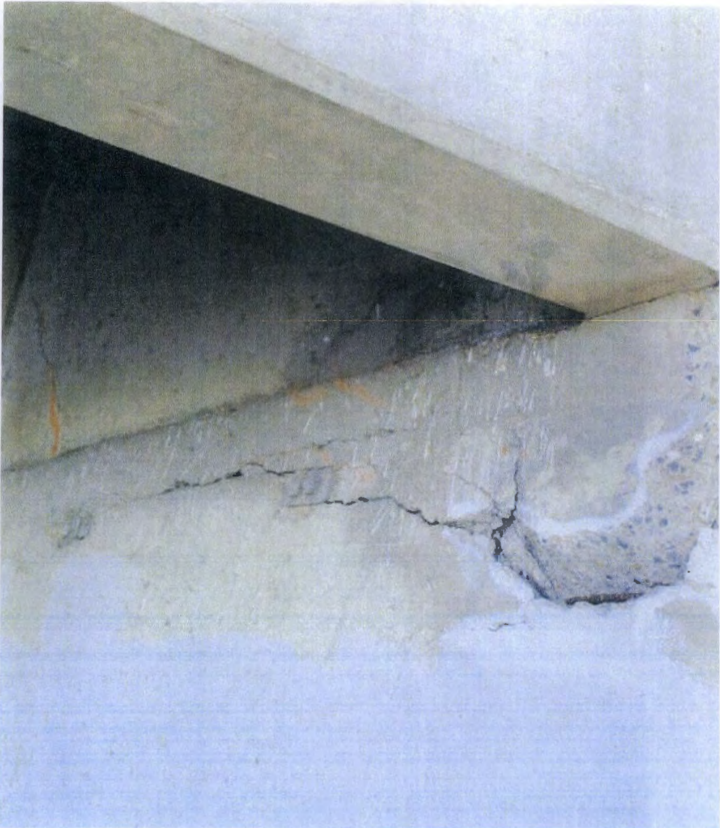
Photo No. 1 Spall at Abutment 1 face under Girder 1.
