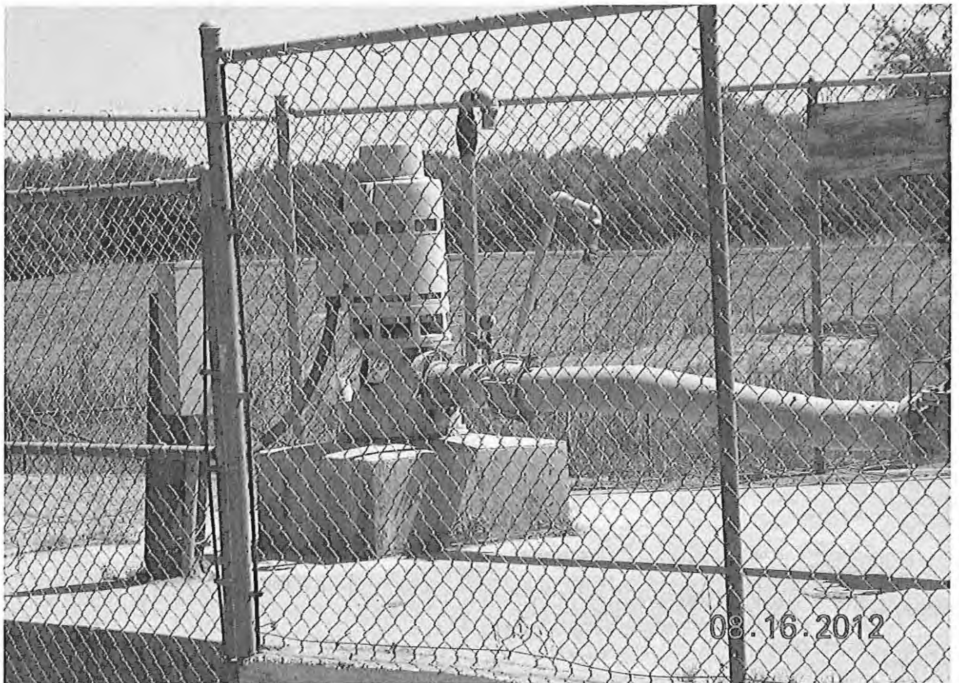
IRRIGATION WELL LAHO PARK
