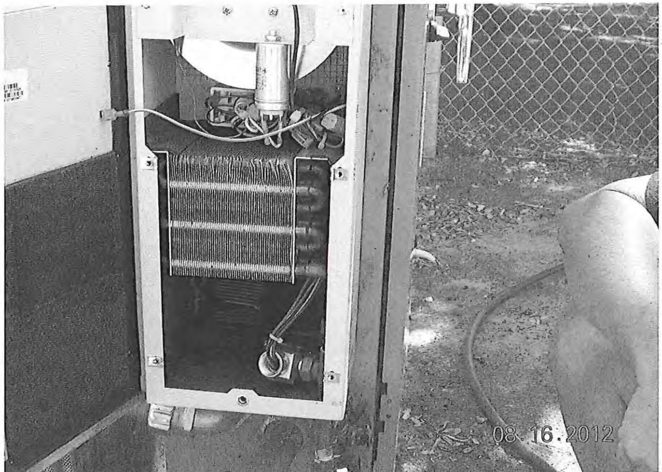
Heat Exchanger Water-Air
