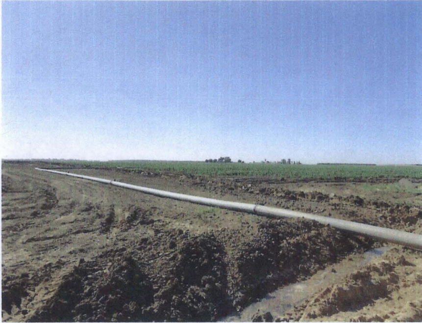
Figure 16. Irrigation line between fields 2 and 3
