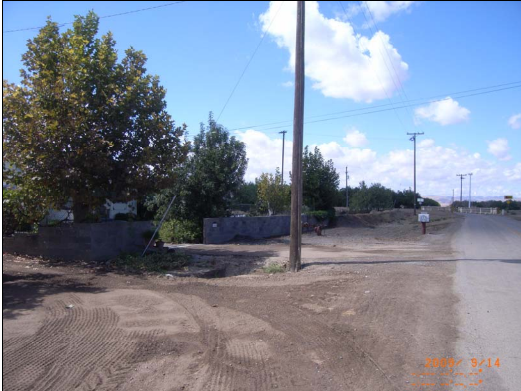
Figure 2-9: Flood Wall Risk Reduction Measure at a Rural Residence near Orestimba Creek
