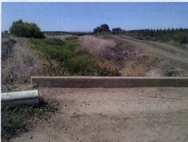
Figure 6. Drainage ditch with major reduction of water-holding capacity due to vegetation and sediment build-up
