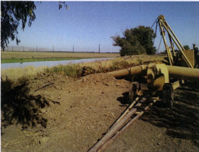
Figure 11. Operator pumping water from field 1&2 into the Marshall Drain
