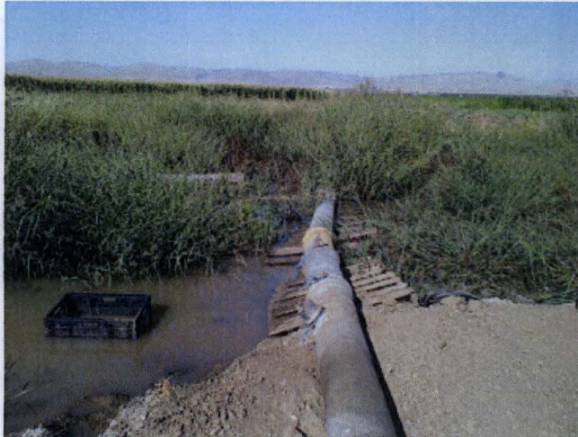
Figure 4. Drainage ditch congested by vegetation, trash, debris
