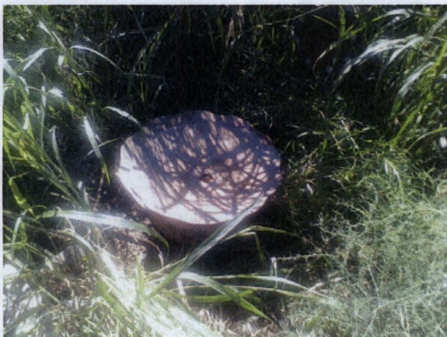
Figure 3. Well 6/8-20C1 in Field 8—Surface water observed draining directly into groundwater through areas where pipe has deteriorated.
