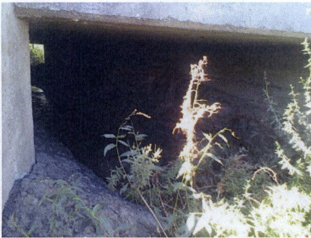
Figure 8. Culvert (same as Figure 7) demonstrating severe sediment build-up
