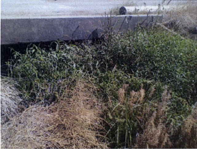
Figure 7. Culvert in-flow obstruction
