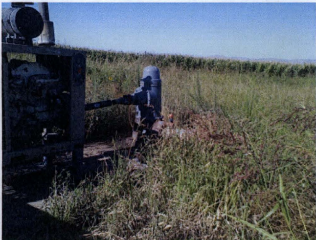
Figure 2. In-use Well in Field 3
