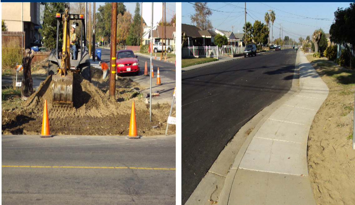
Photos reflect before and after work in downtown residential streets lacking curb, gutter, storm drain, sidewalks, and ADA ramps in Ceres.
