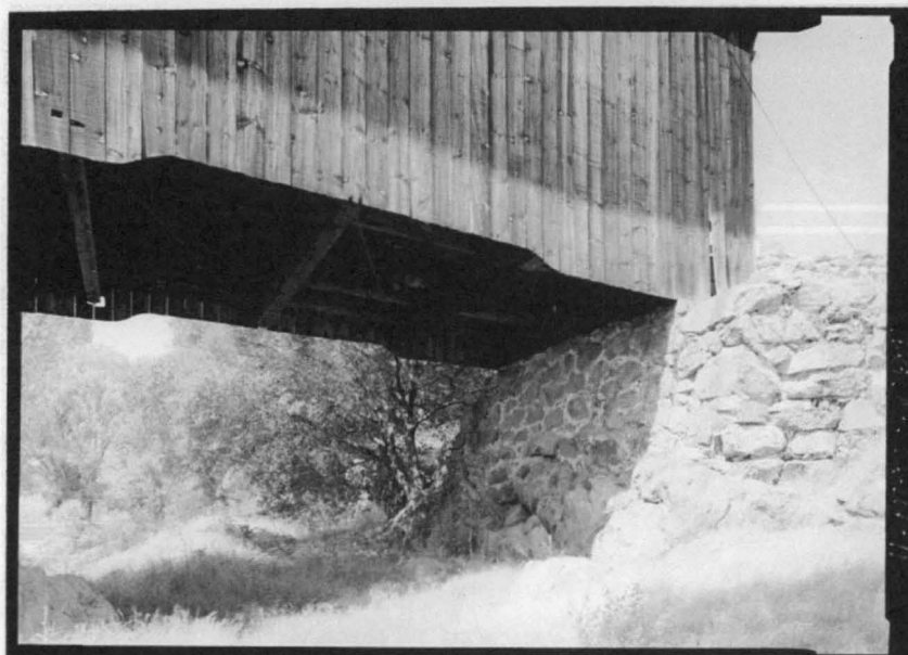
KNIGHT'S FERRY BRIDGE. Floor system detail at northwest abutment. Photograph by Jet Lowe, 2004 [HAER No. CA-314-11]
