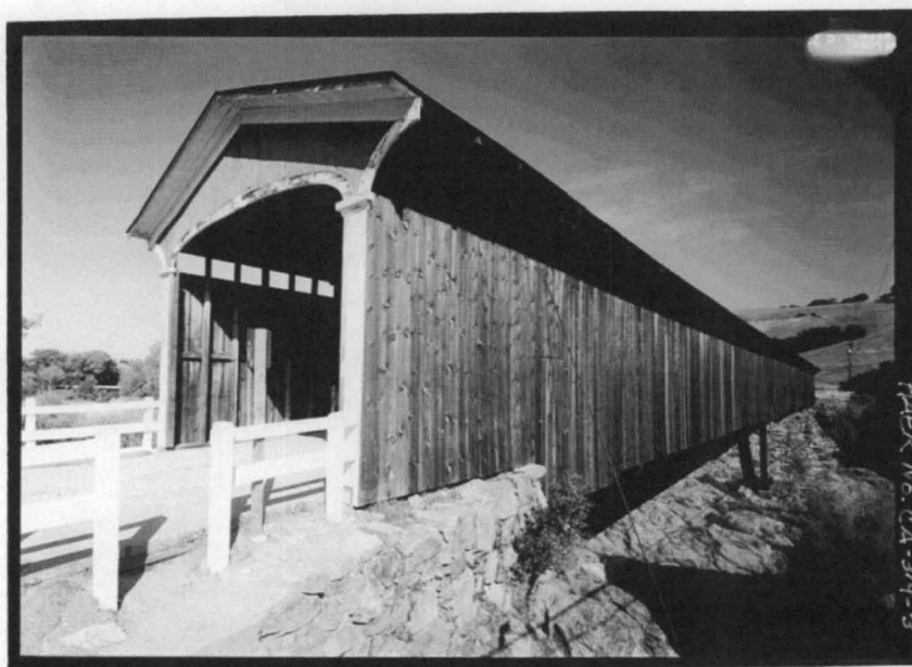
KNIGHT'S FERRY BRIDGE. Oblique perspective from southeast portal. Photograph by Jet Lowe, 2004 [HAER No. CA-314-3]
