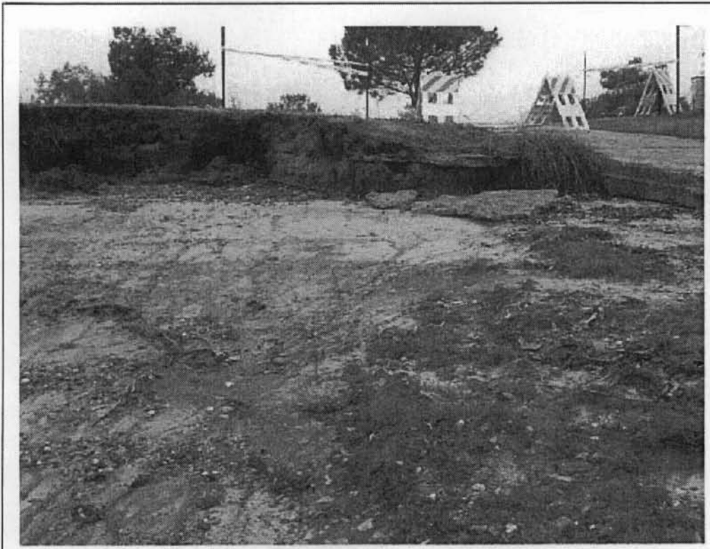
Erosion along the bank adjacent to the existing boat ramp, looking southwest; 01/07/09.
