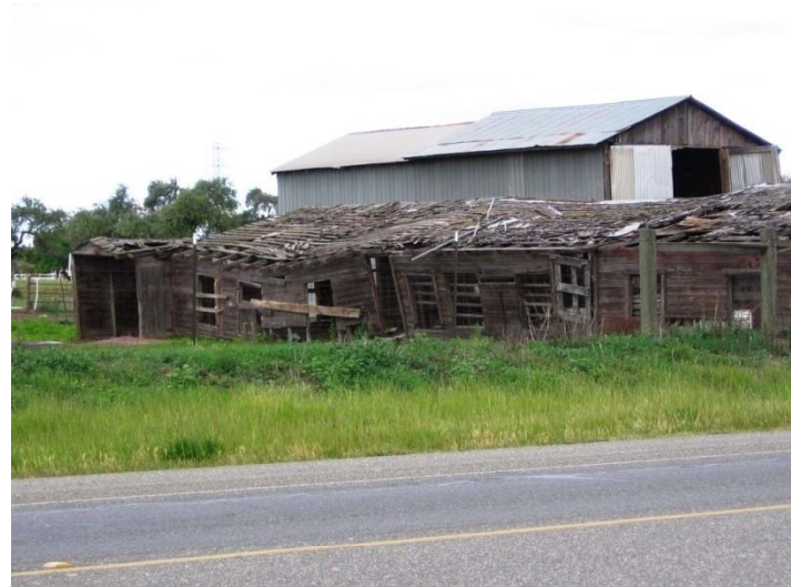
Seriously damaged and deteriorated building
