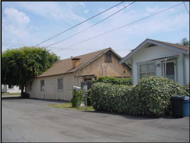
OV – Overgrown/Hazardous Vegetation
