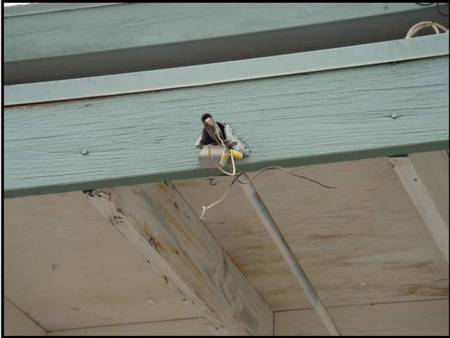
AEH – Apparent Electrical Hazards
