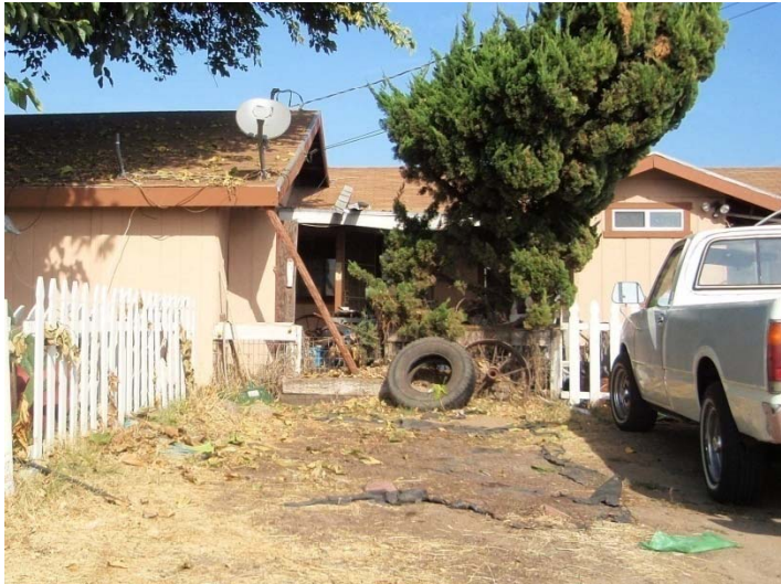
Damaged roof; dirt driveway; bare plywood used as building material
