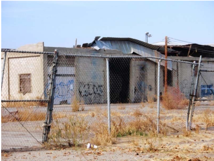
Vacant building; serious damage and deterioration; graffiti; damaged chain link fence; weeds
