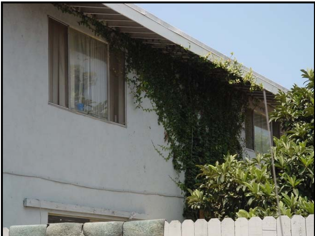
OV – Overgrown/Hazardous Vegetation
