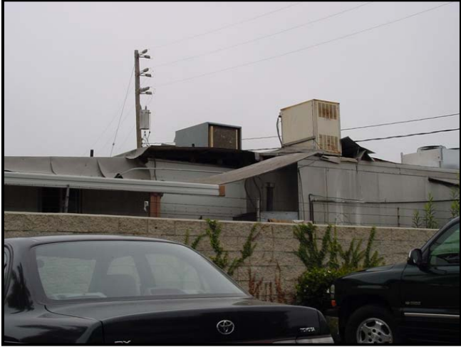
FME – Deteriorated Fixtures/Mechanical Equipment/HVAC
