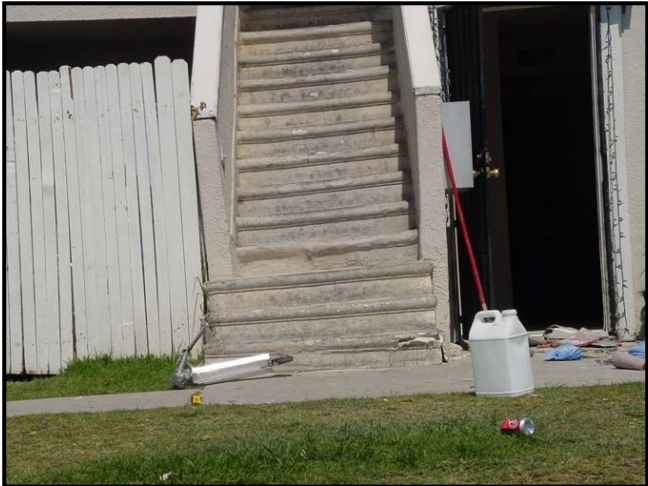
UST – Unsafe Missing Stairways or Walkways
