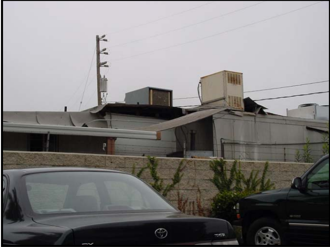
FCM – Faulty Construction Materials
