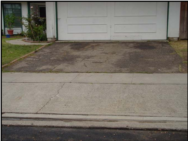
PRI – Deteriorated/Absent Private Infrastructure
