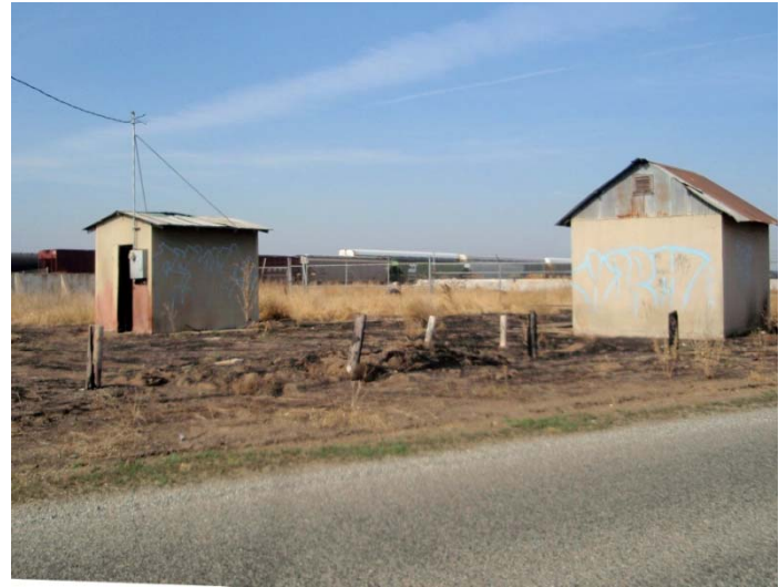
Vacant buildings; serious damage and deterioration; graffiti; weeds
