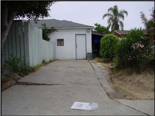
GC – Garage Conversion Not Permitted
