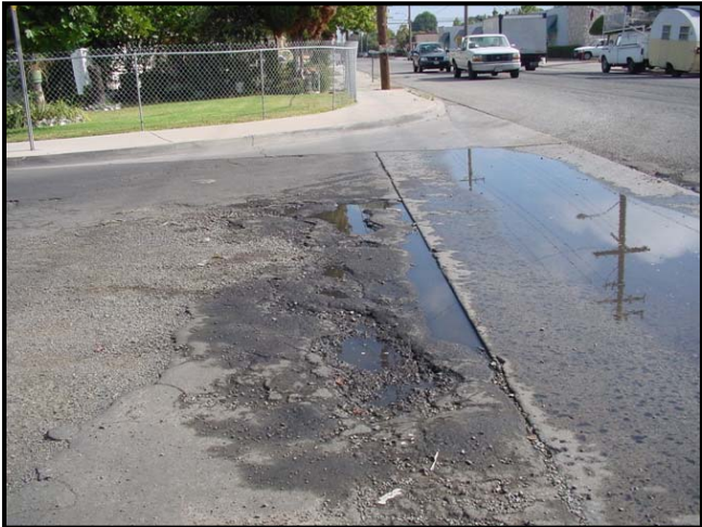
PUI – Deteriorated/Absent Public Infrastructure Street, Curb, Parking
