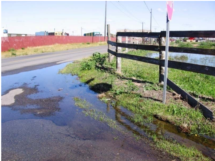
No curb, gutter, or sidewalk; flooding; damaged fence
