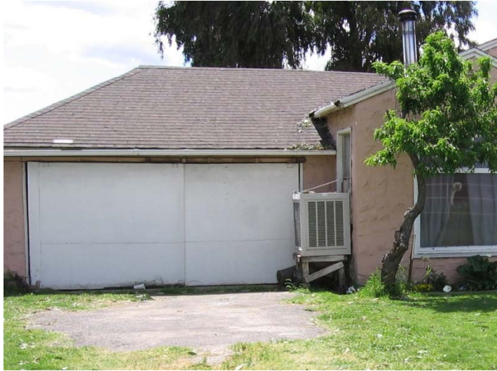
Inadequate and damaged support for mechanical fixture; blocked garage door; damaged driveway
