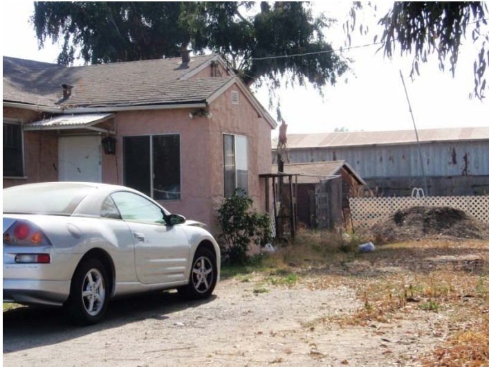
Poorly patched exterior wall repair; deteriorated secondary structure; damaged and rusted building; dirt driveway
