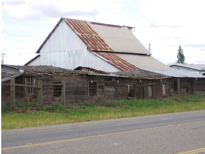
Seriously damaged and deteriorated buildings
