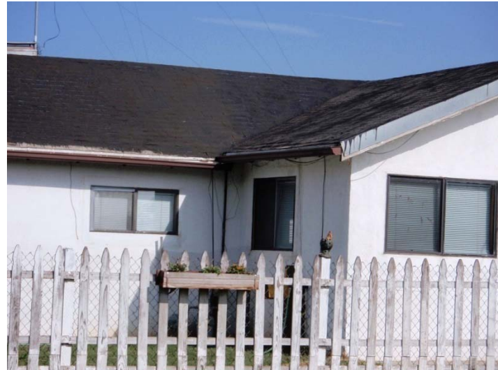
Damaged roof and apparent electrical hazards with loose and exposed wiring
