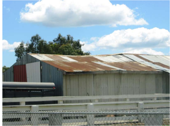
Seriously damaged and deteriorated building
