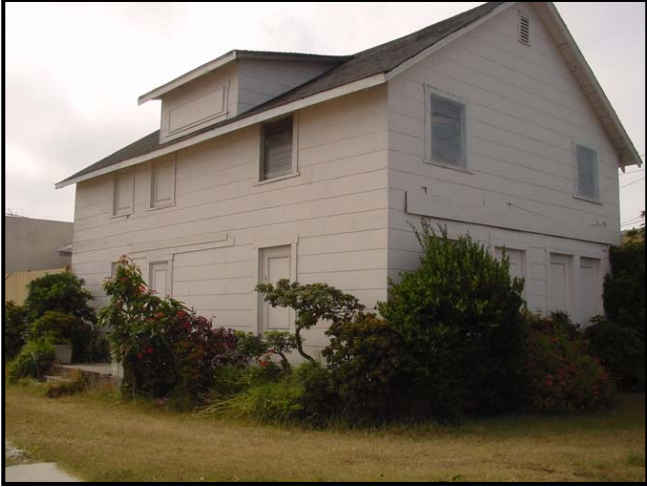
BU – Boarded Unoccupied
