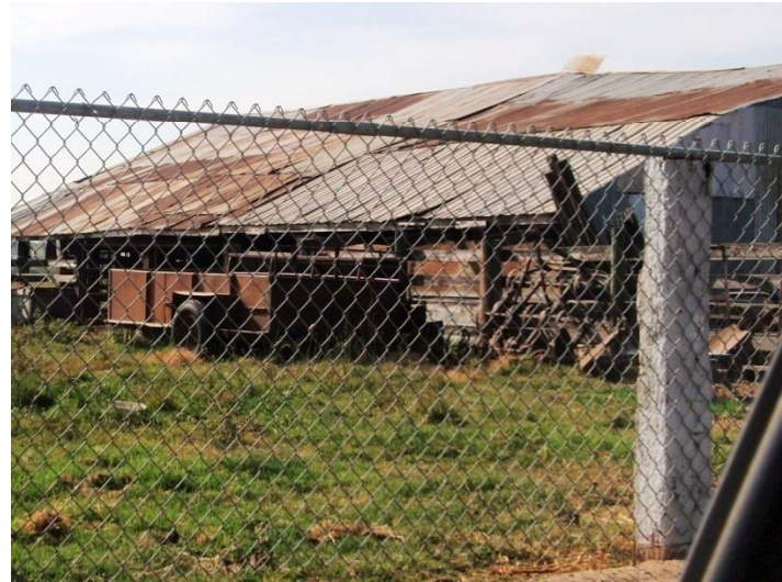
Seriously damaged and deteriorated building
