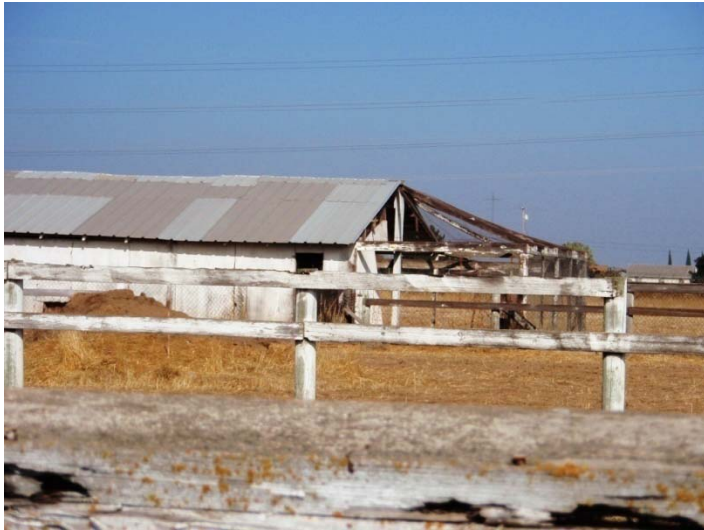
Serious damage and deterioration
