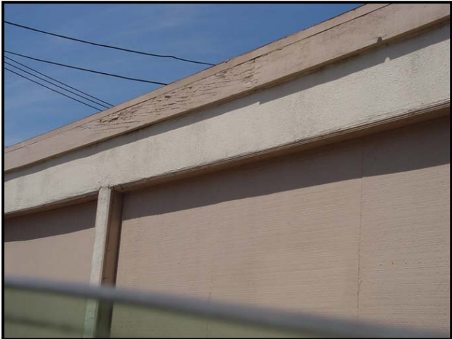
P – Paint-related issues
