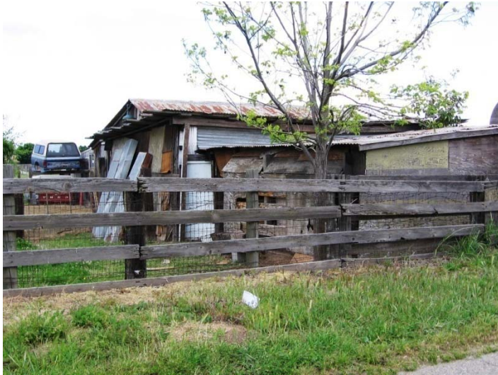
Seriously damaged and deteriorated building; inadequate building materials
