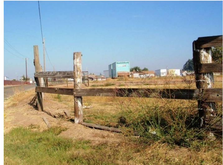
No curb, gutter, or sidewalk; damaged fence; inoperable vehicles; overhead utility lines
