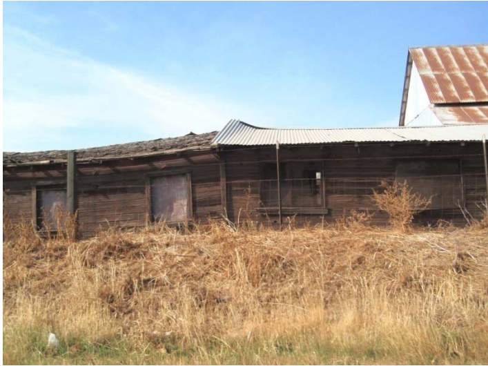
Seriously damaged and deteriorated building; weeds
