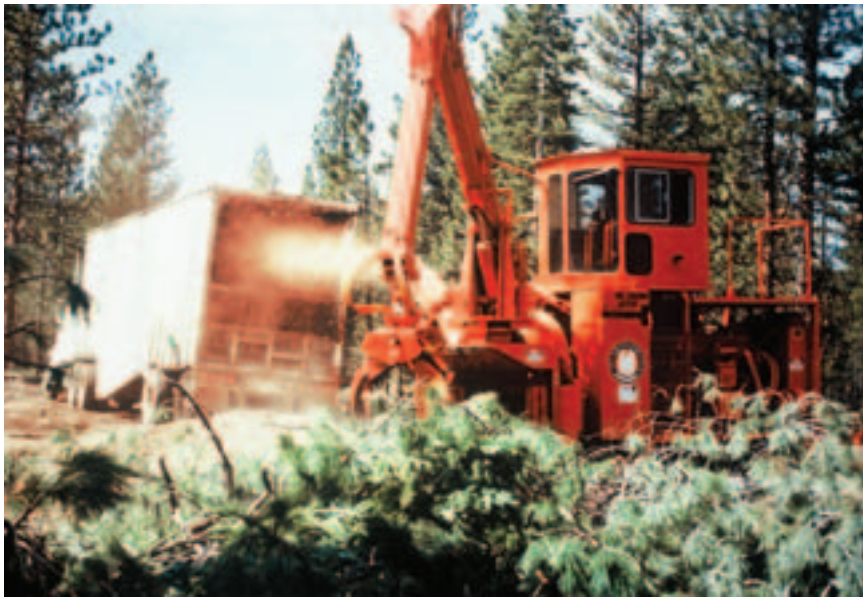
Biomass materials must be chipped in the forest and transported to biomass power plants. Each chip van contains enough fuel to power one home for about 250 hours.
