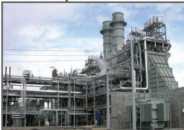
Walnut Energy Center began operation on February 28, 2006. The plant has a total generating capacity of 250 megawatts.
